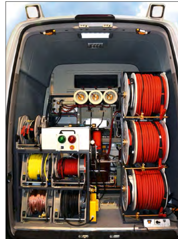
Rear View of the HV compartment
